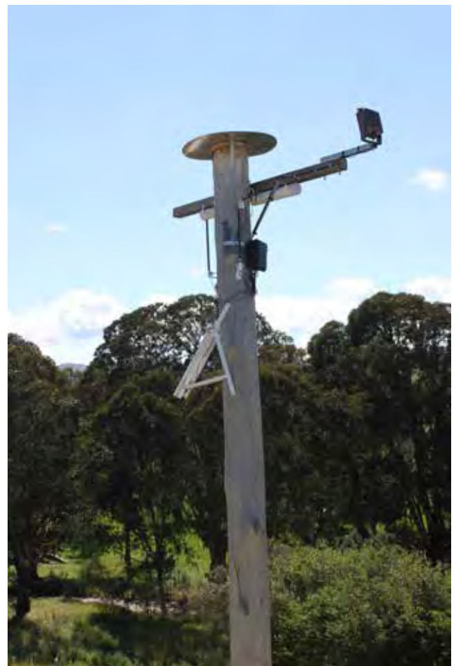
Glider poles are installed on the verges of linear infrastructure or in the centre median at locations where the size of the gap in tree cover exceeds the glide distance of gliding animals. This close-up shows the cross-arm or launch platform at the top of a glider pole, along with cameras and solar panels to evaluate use. The metal shield on top of the pole and the pipe under the cross arm provides shelter from aerial predators. The cross-arm points towards the trees on the opposite side of the infrastructure, thereby decreasing the size of the gap to be crossed. © Rodney van der Ree
