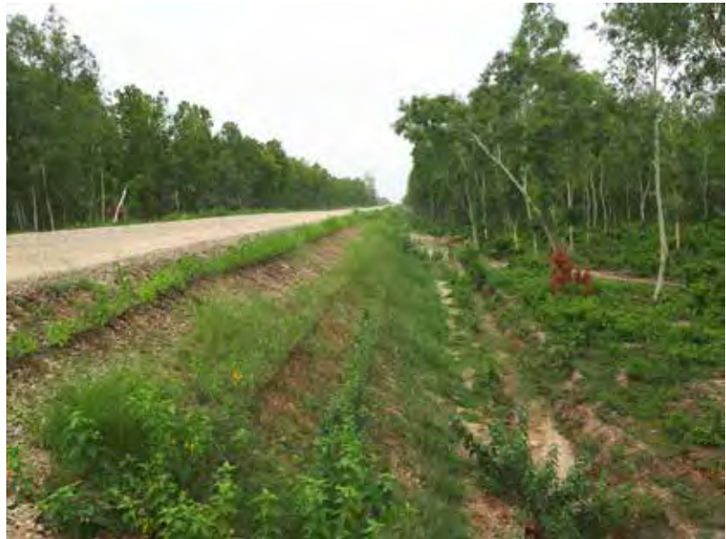
Roadside grading with revegetation after construction, part of a revised mitigation strategy for the Narayanghat – Butwal (NB) Road, Nepal © Pramod Neupane
