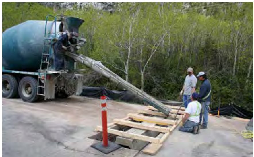
Construction of a salamander-friendly underpass tunnel in Waterton Lakes National Park, Alberta, Canada. © Cyndi Smith, Parks Canada
