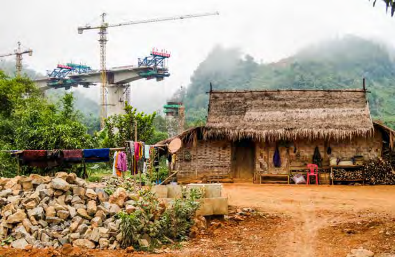
Construction of the 414 km Laos - China high speed railway brings infrastructure prominently in view of a rural home in Laos. The rail cuts through 167 Laos villages, and research has shown that many people in the affected villages were unclear about plans, timelines, land compensation processes and the ability to comment on construction. © Jessica DiCarlo
