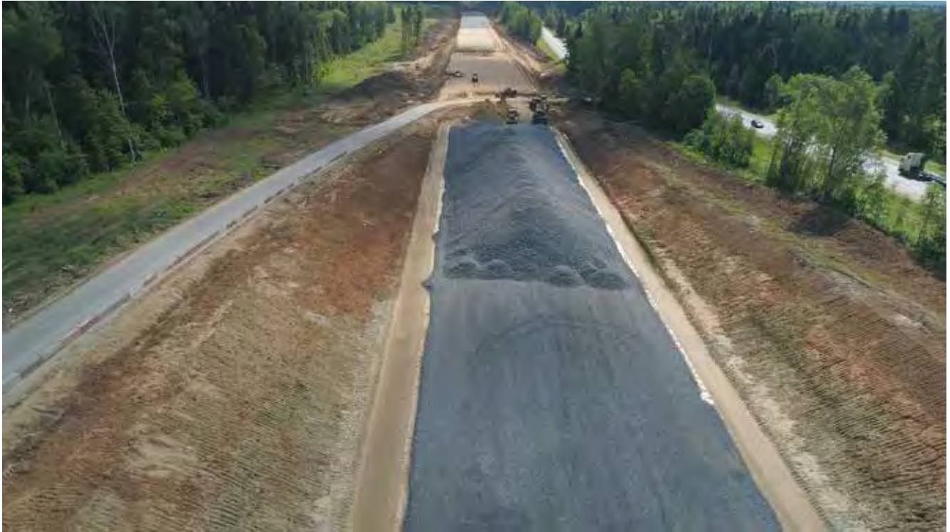
Construction of a toll road through a rural area, intended to replace an existing road © Alex Traveler / Adobe Stock
