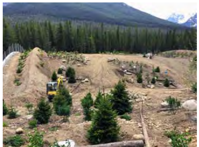
Overpass construction in progress that includes natural surfaces, vegetation variations and design elements to reduce noise and light disturbances to provide favourable conditions for a diversity of species to cross the Trans-Canada Highway, Banff National Park, Alberta, Canada. © Terry McGuire
