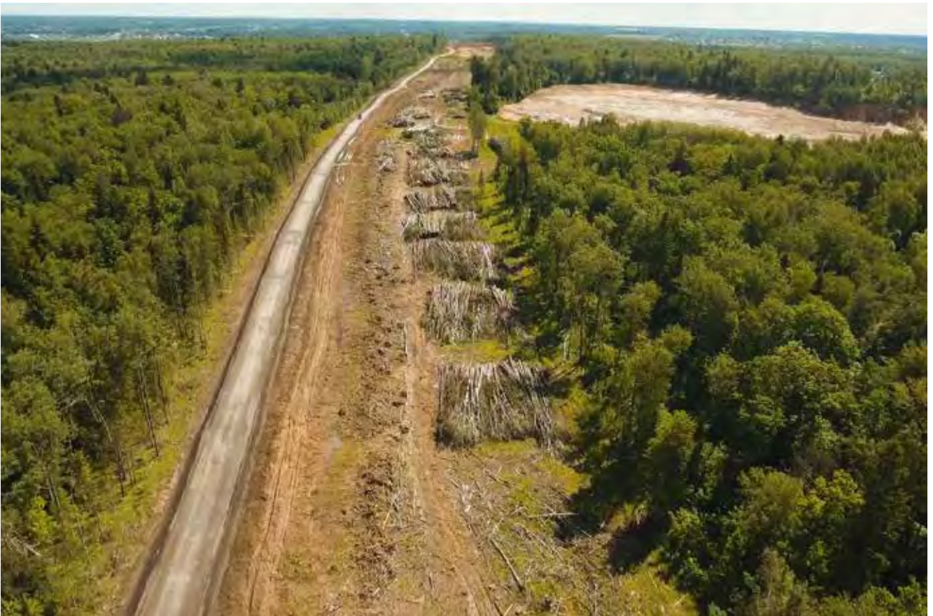
Forest clearing for construction of a toll road through rural land. The amount of land that needs to be cleared for infrastructure projects is often much wider than the roads, rails, or canals themselves. © Alex Traveler/ Adobe Stock
