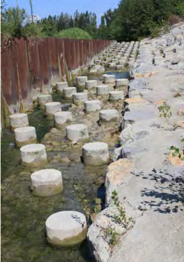
Fish ladder on the Roubion River near Lyon, France. This structure was built in 2011 to provide passage for fish around a weir in place since 1964, originally built to protect downstream infrastructure from flood damage. The ladder and ledges were designed for eels, numerous fish and beaver. © Rodney van der Ree
