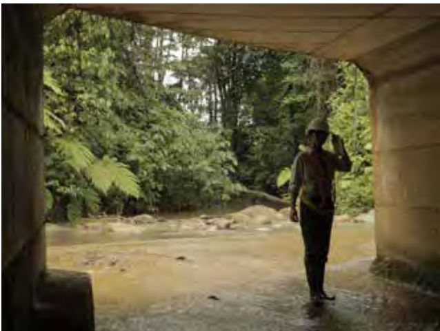
A technician stands in a highway underpass incorporating design for free stream flow and ledges for dry passage by wildlife. © Daniela Araya-Gamboa/ Panthera
