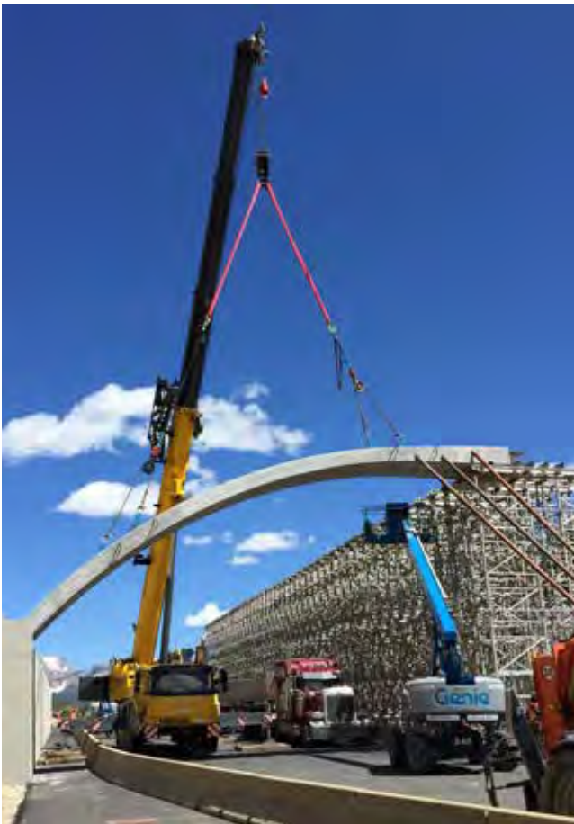
Construction of an overpass over Interstate 90 on Snoqualmie Pass, Washington, USA. Spanning six lanes of traffic, this large overpass is just one piece of a multi-phase, multi-decade effort to restore connectivity in the Cascade Range. Other elements include a 330 m elevated stretch where wetlands and creeks flow beneath the highway, and numerous expanded culverts. Monitoring has documented around 4,000 successful wildlife crossings per year. © Terry McGuire
