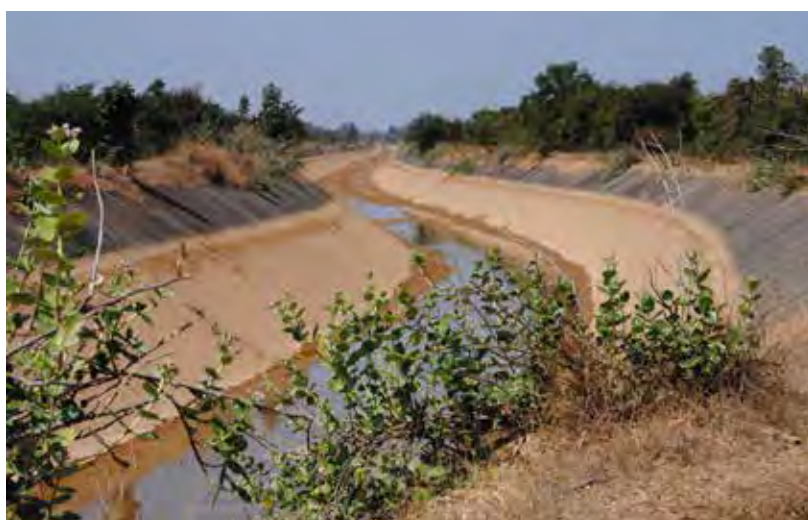
Top: Egress steps next to a wildlife crossing structure over a canal in central India. Middle: Sediment from canal water has partially filled many of the lower steps. Bottom: An unmitigated portion of the same canal © Robert Ament
